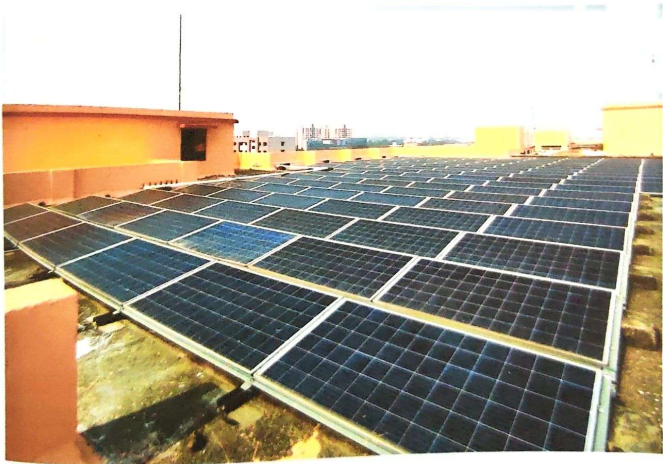
SOLAR PANEL INSTALLED ON THE ROOF TOP OF THE ARTS BLOCK
