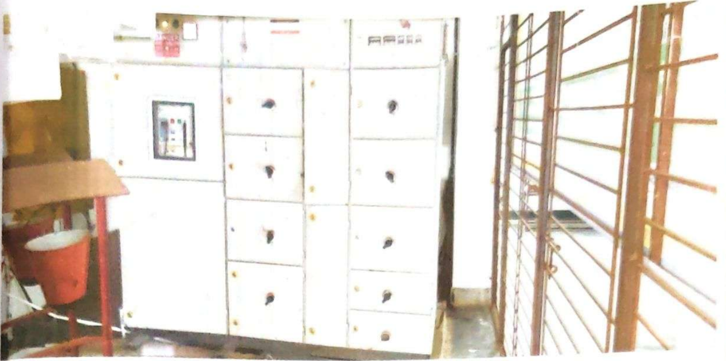
PANEL SWITCH (ARTS BLOCK)
