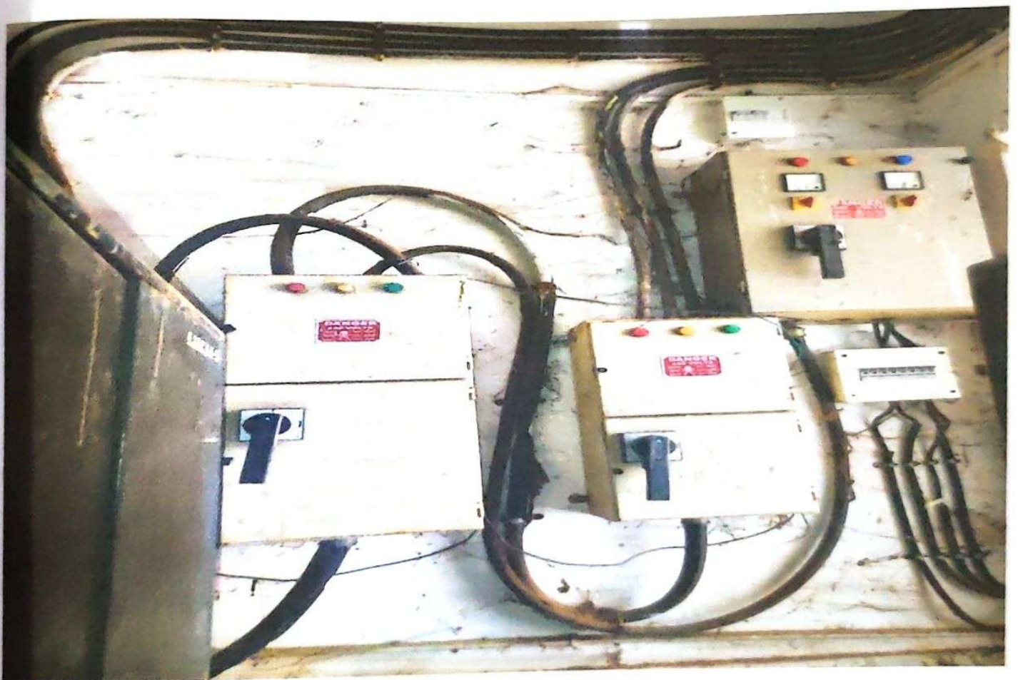
MAIN SWITCH & PANEL (ADMINISTRATIVE BLOCK)
